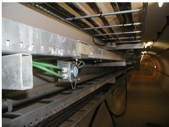
Junction box with signal cabling in ARC
