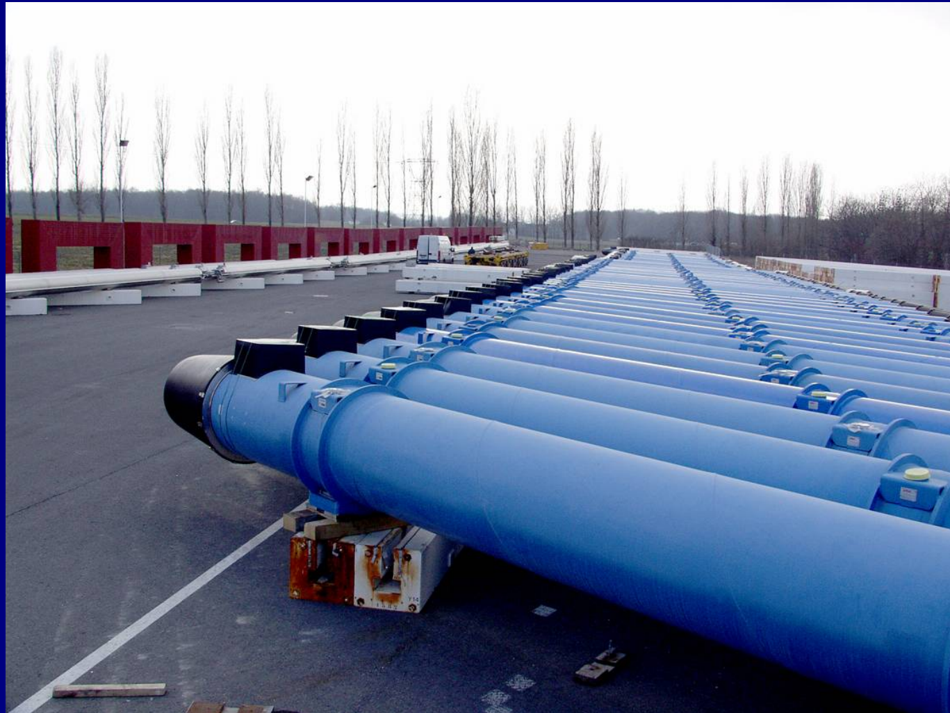
waiting to be installed in the tunnel
