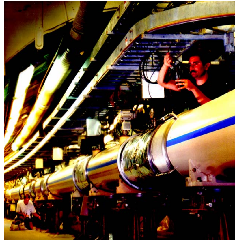
the RHIC tunnel
