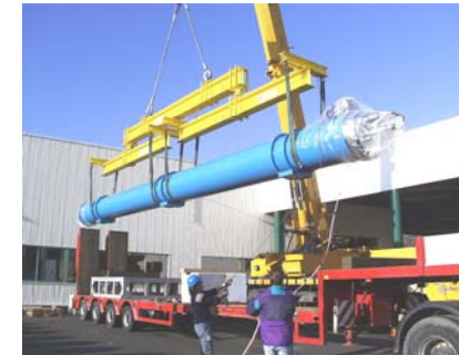
Unloading a 27 tons dipole
